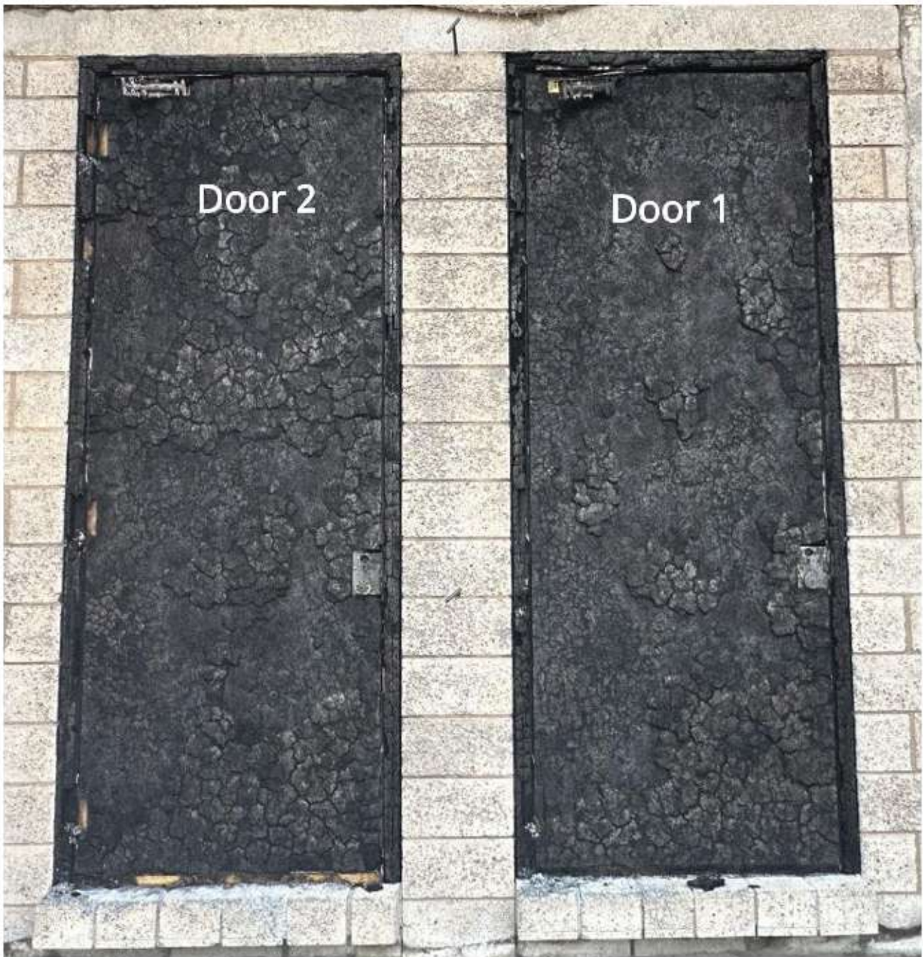
Photo 9. After the Hose Stream Test.
